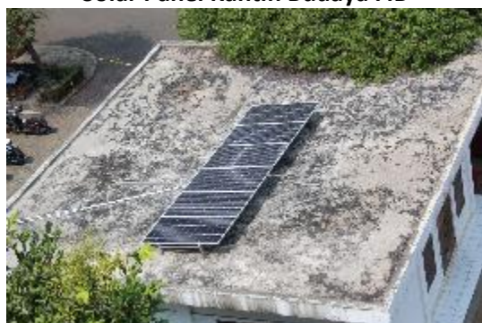
Solar Panel gedung X (Ruang genset)
