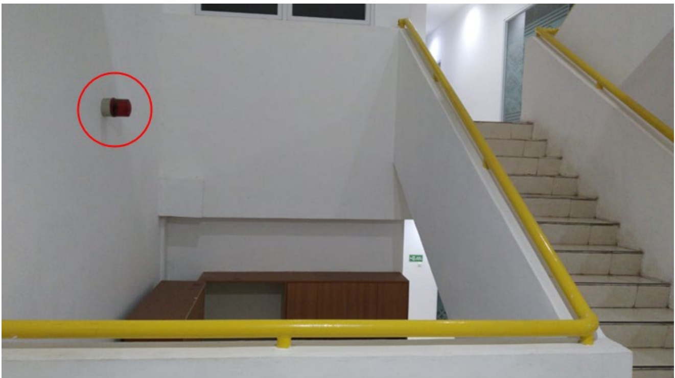
Smoke detector alarm
