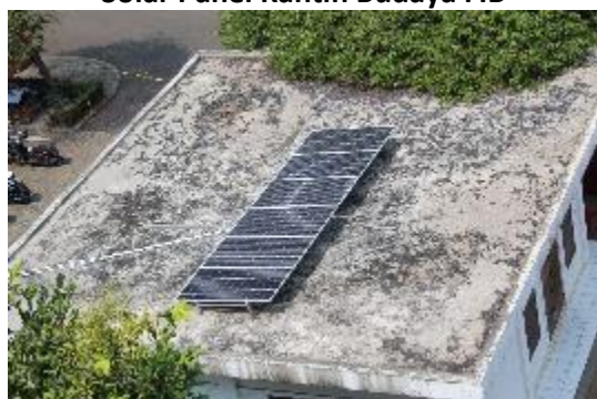
Solar Panel gedung X (Ruang genset)
