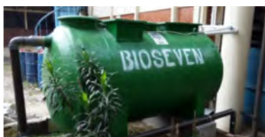
Gambar 6.8 IPAL Mengolah Limbah Beracun Sebelum Dibuang Figure 6.8 WWTP Processes Toxic Waste Before Disposal
