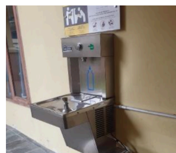
Gambar 6.5 Drinking Fountain di Asrama Figure 6.5 Drinking Fountain at the Dormitory
