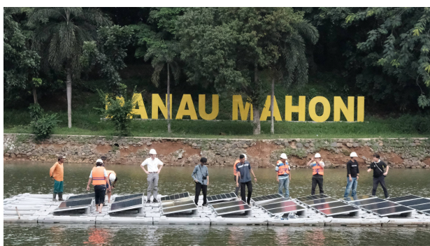
Gambar 7.1 PLTS Terapung Bifacial Figure 7.1 Floating Bifacial Solar Power Plant
